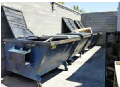
Current state of OC trash service area is unsightly and requires seven days-per-week dumpster service; compactors will save money over time and allow cardboard recycling
